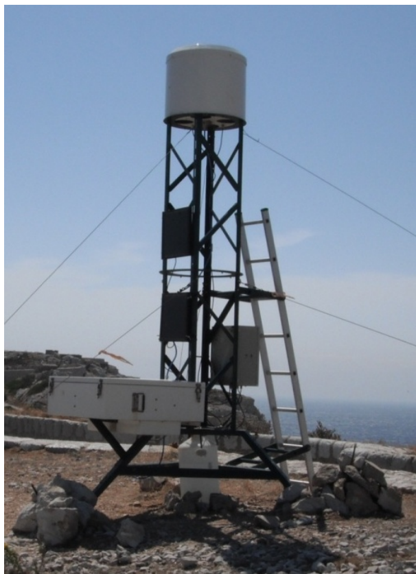
Figure 1. The CARAGA collector operating on Frioul Island.
