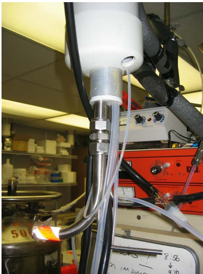
Figure S3. Multiple conditioned sample lines from the roof as they enter the laboratory immediately below the chamber.
